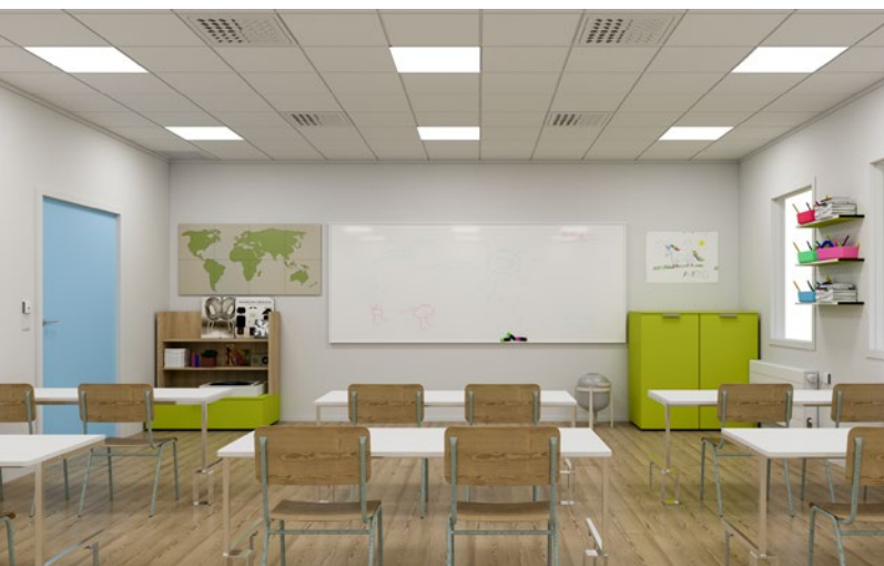
Classroom with demand-controlled air regulation, occupancy sensors and control of radiators.
