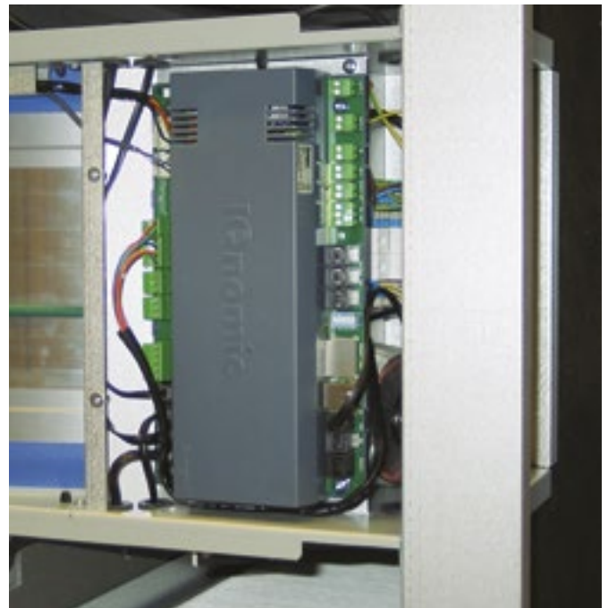
IQnomic control unit
